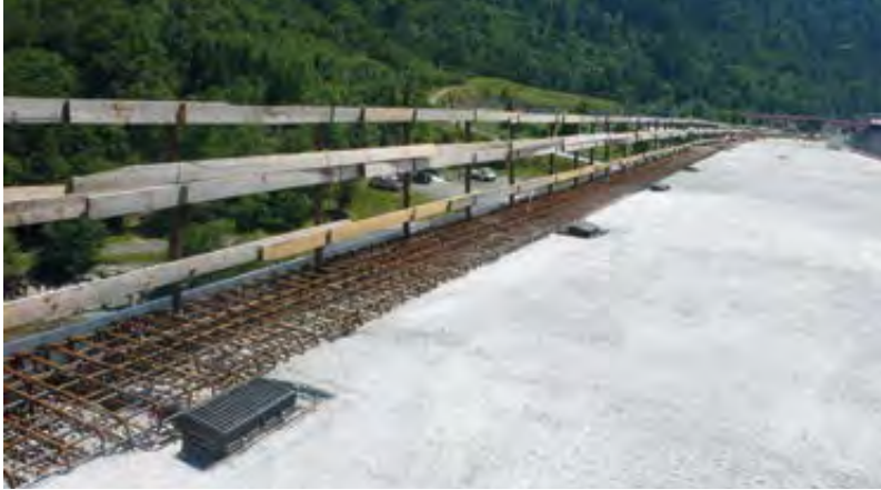
Bridgedrain - Cuneo (CN)
